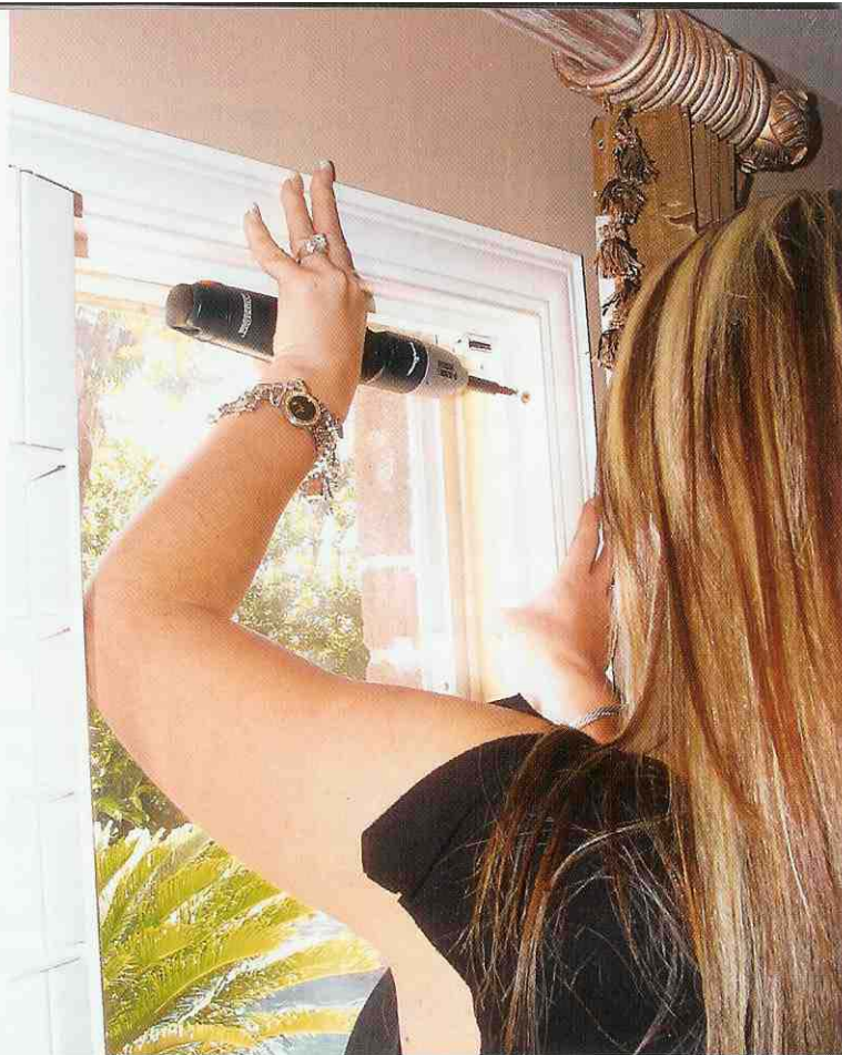
Homeowners simply screw in four to eight pre-drilled holes to mount the Pro Décor Shutter. J & L Distributors can provide measurement and installation for homeowners, decorators and builders.
